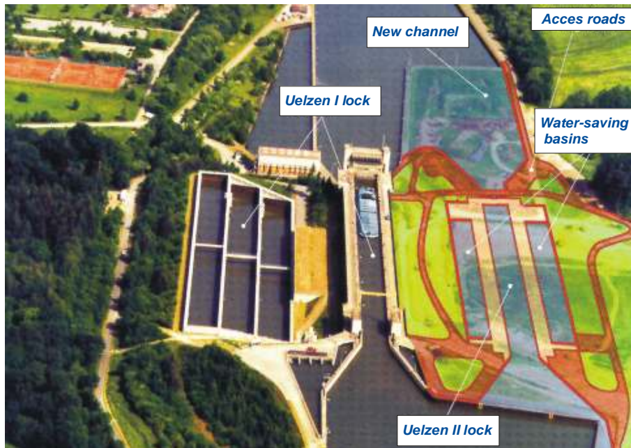
Fig. 1: Aerial view of the existing Uelzen I lock and the new Uelzen II lock (under construction)
